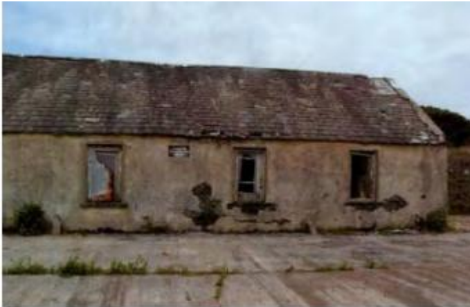
Plate 14-6: RPS 637 (photo courtesy of RPS, Vol 4 CCDP).
